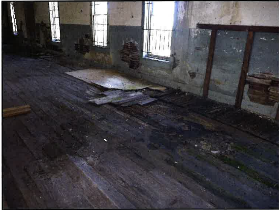
Photo 5 – Second floor damage due to water intrusion.
