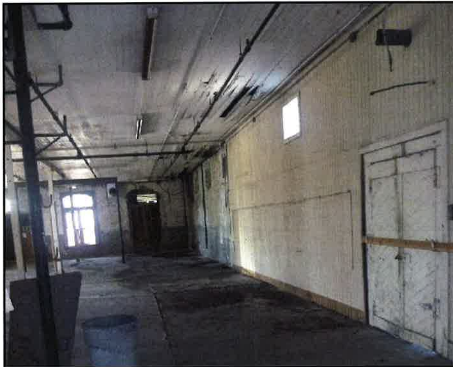
Photo 4 – Wider view of first floor with ceiling damage.
