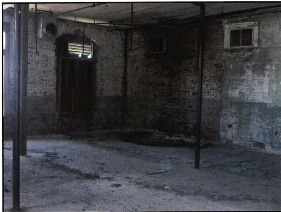
Photo 2 – First floor showing ceiling damage and where water has pooled.
