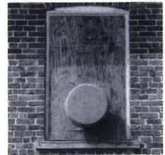
c. The exhaust fan has tamper-proof housing.
