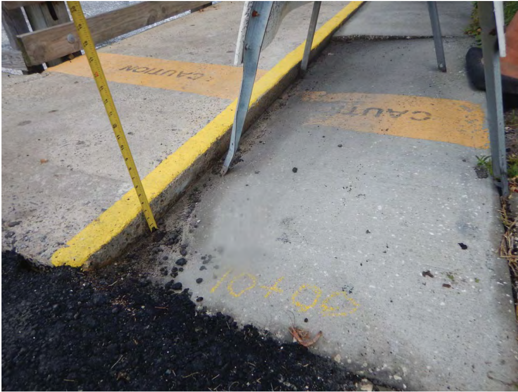
Photo 11 –Typical Settlement behind Concrete Seawall
