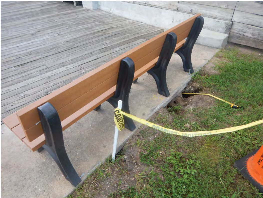
Photo 12 – Typical Voids/Undermining behind Concrete Seawall
