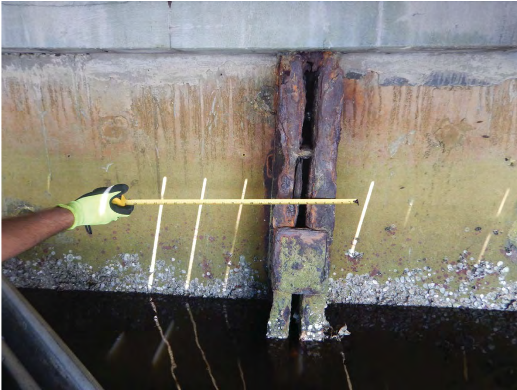
Photo 15 – Typical Heavy Section Loss on Steel Channel Supports for Concrete Seawall
