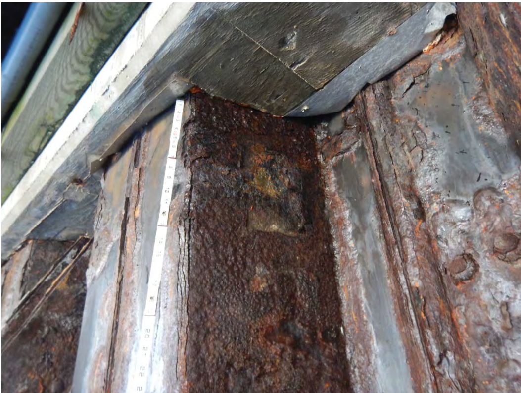
Photo 20 – Area of Maximum Section Loss for Steel Sheet Pile Wall
