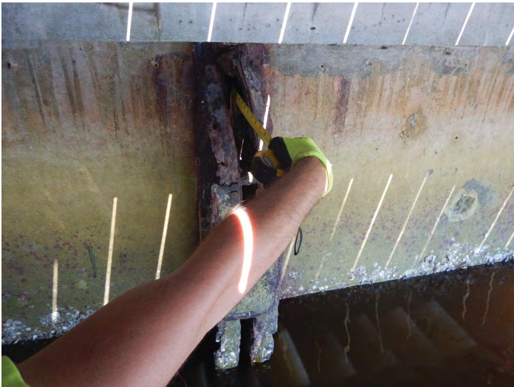
Photo 16 – Typical Heavy Section Loss on Steel Channel Supports for Concrete Seawall
