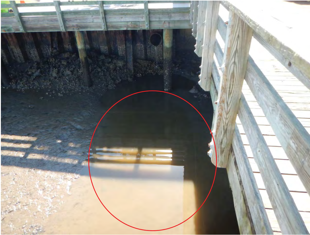
Photo 17 – Local Scour at Drainage Pipe Penetration in Steel Sheet Pile Wall
