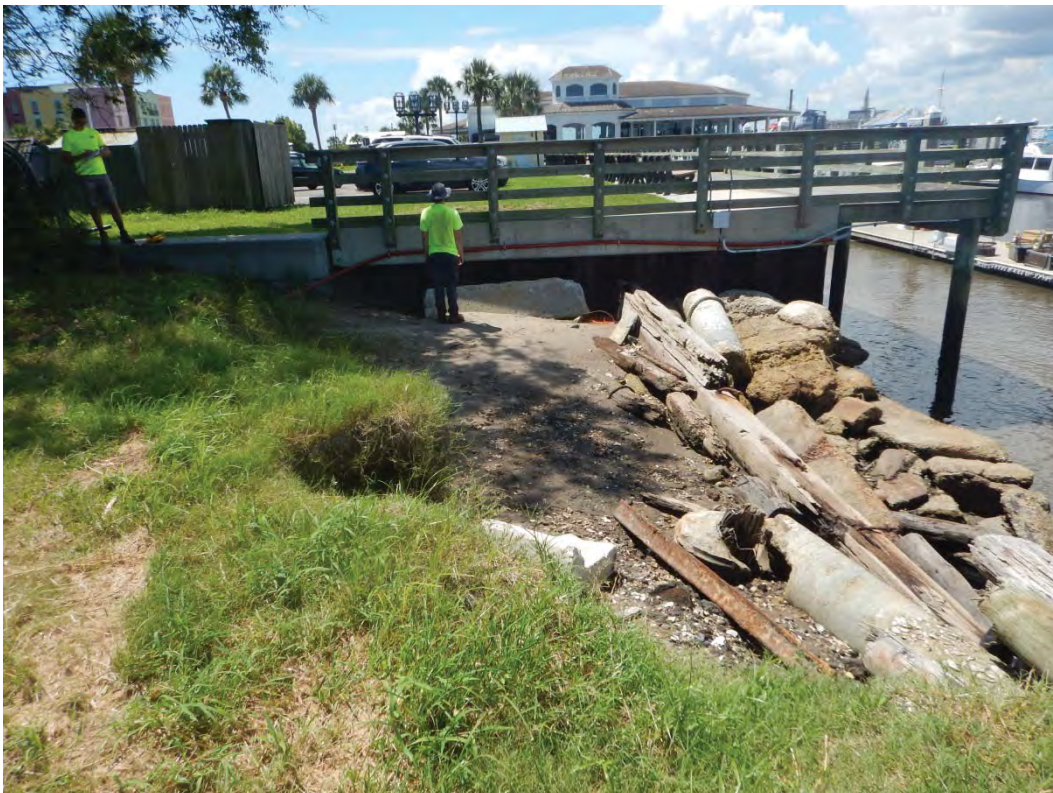
Photo 18 – Local Scour at Steel Sheet Pile Wall Extension
