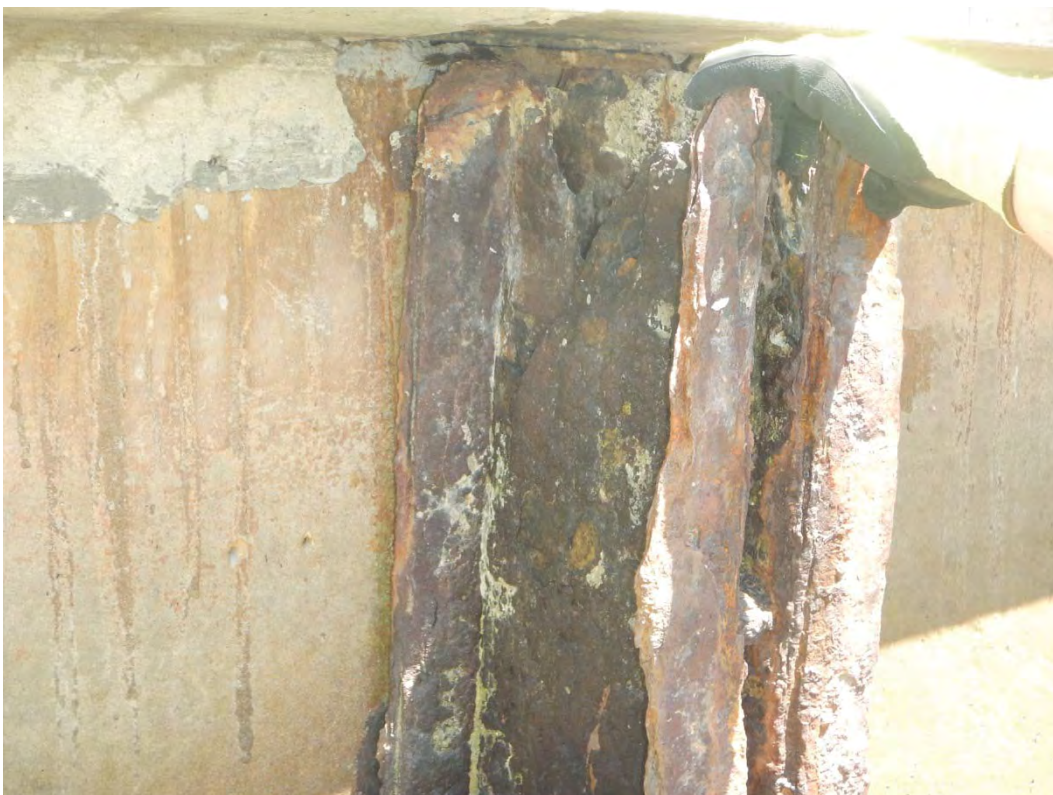
Photo 14 – Typical Heavy Section Loss on Steel Channel Supports for Concrete Seawall
