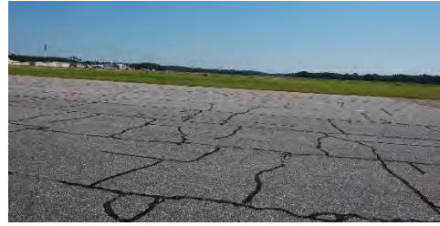
Photo 3. Abandoned runway with deteriorating surface.
