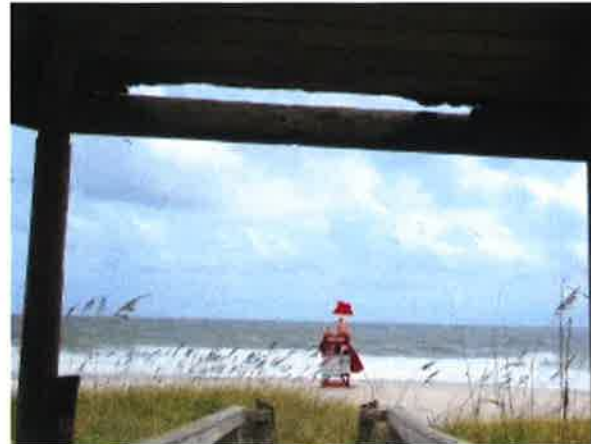
VIEW OF THE OCEAN AND DETERIORATED ROOF OF SOUTHERNMOST GAZEBO AT MAIN BEACH
