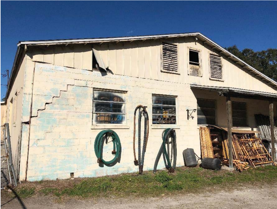
Figure 1 – Cracks near southwest corner of building at 400 south 8 th Street.
