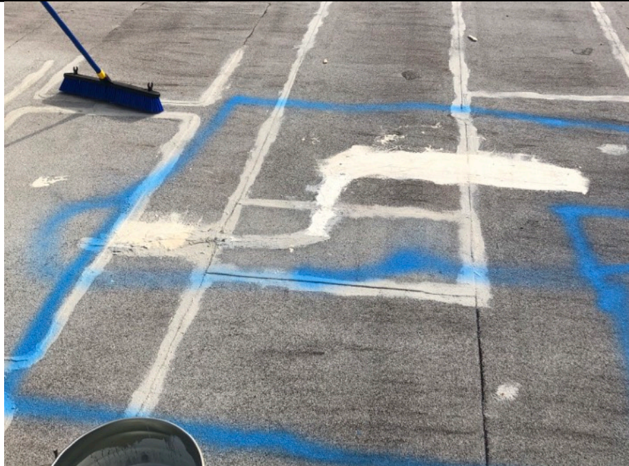
Overview of split membrane caused by lack of expansion joint.
