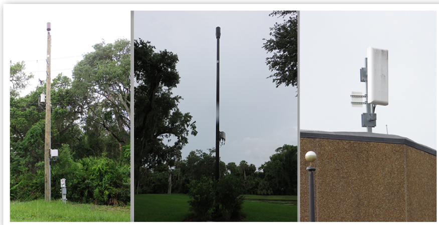
Figure 6: Non-Concealed Small Cell Base Stations
