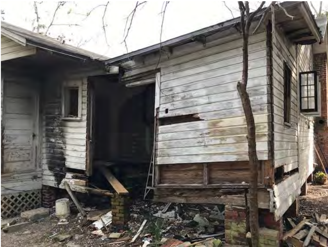
Photo 1: Collapsed Bedroom at Rear of House
