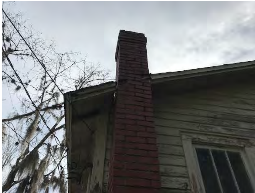
Photo 10: Roof at Chimney in need of repair
