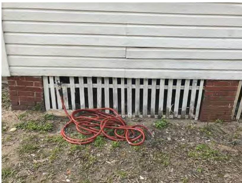
Figure 1Photo 11: Lattice work in need of repair/renovation
