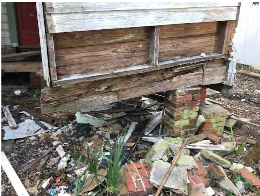
Photo 5: perimeter Beam and Corner Pier Failure
