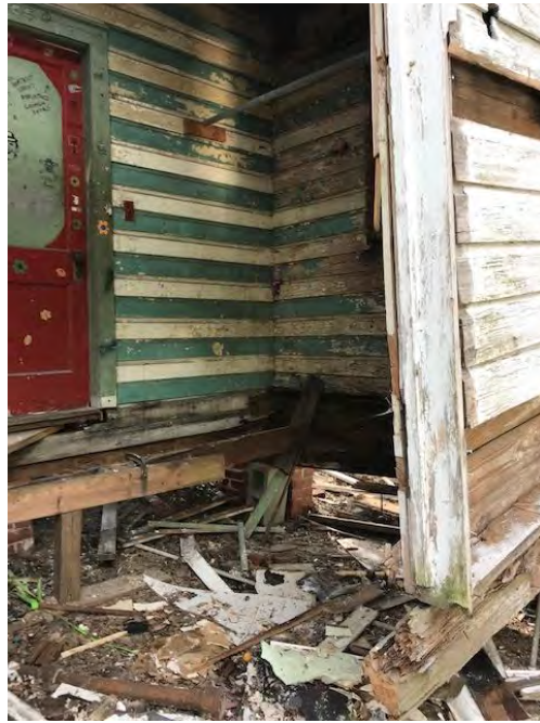
Photo 6: Interior Bedroom Floor Collapse
