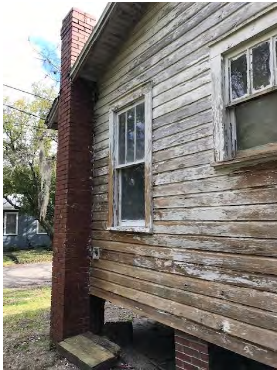
Photo 9: Siding and Trim in need of renovation/repair
