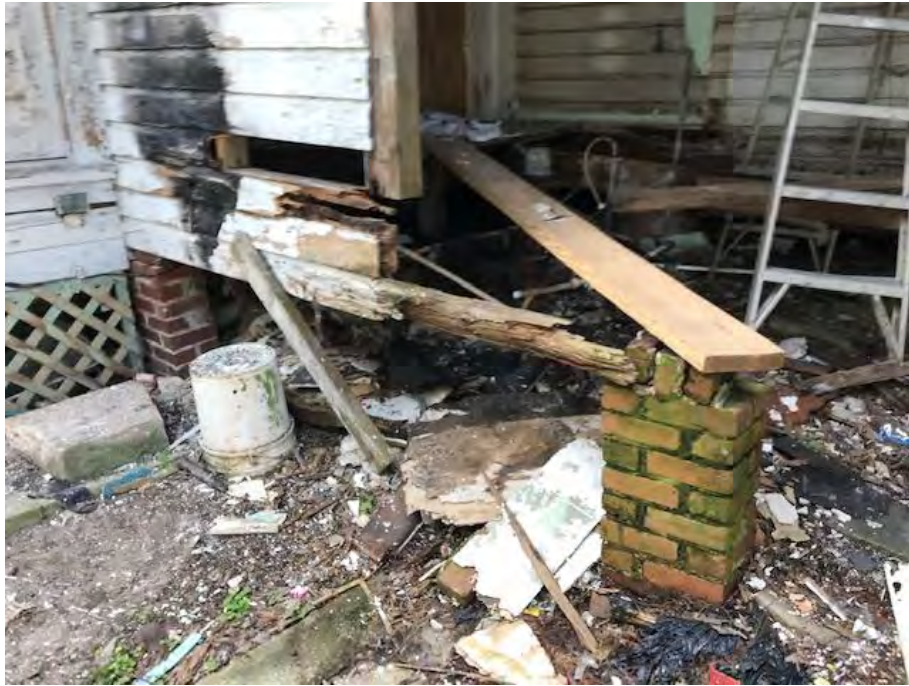
Photo 4: Perimeter Beam and Center Pier Failure
