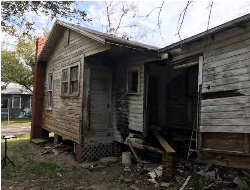
Photo 2: Failed Roof at Collapsed Bedroom
