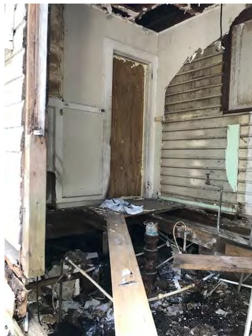
Photo 7: Interior Bedroom Floor Collapse
