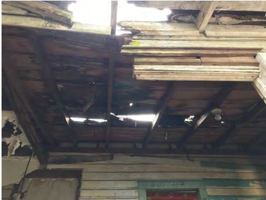
Photo 8: Bedroom Ceiling Failure
