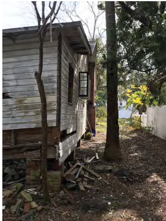
Photo3: Corner Pier Failure
