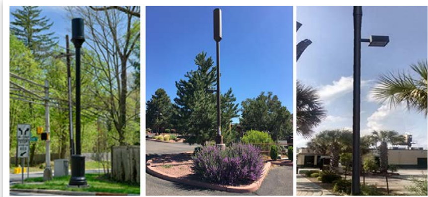
Figure 5: Concealed Small Cell Towers
