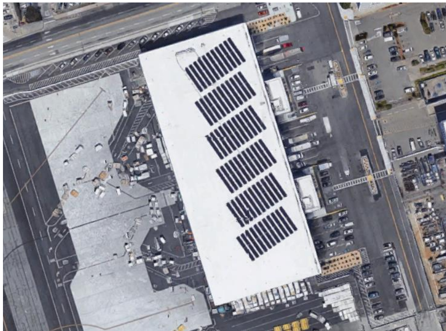
Figure 16 – Rooftop PV array on SFO cargo facility
