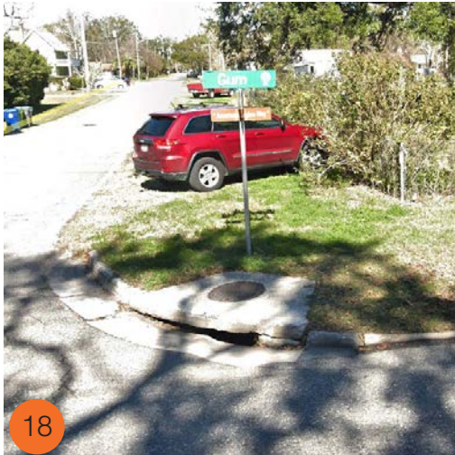
INLET DRAINS THE TRAIL WOULD GO OVER
