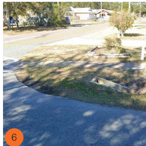
15TH ST. CULVERT THAT WILL REQUIRE REALIGNMENT
