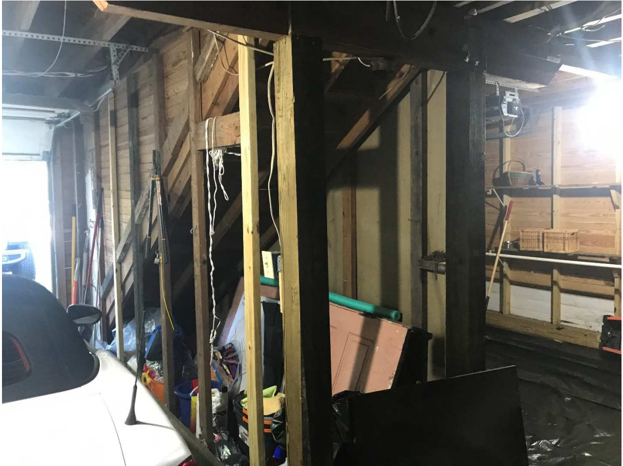
Garage interior showing framing and replacement framing due to rot.
