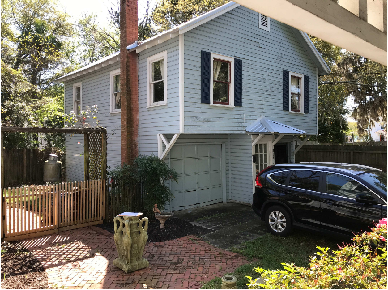
Outbuilding photo showing low lying condition of building and rot from water damage visible at door.
