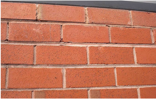
Photo 1 Mortar Joints in Need of Repointing
