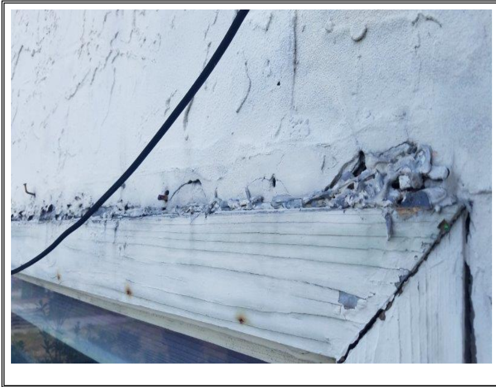
PHOTO 20: Sample 120: Exterior Window Frame Sealant.
