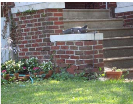
Brick Piers with Missing Mortar
