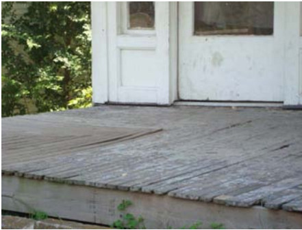
Sagging Porch Floor
