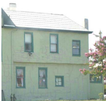
Poorly Patched Cracks on a Stucco Home
