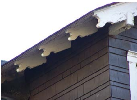
Exposed Rafter Tails
