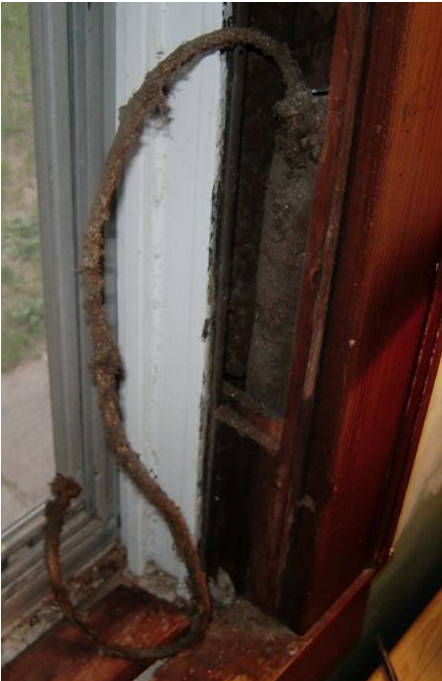
Broken Sash Cord and Weight
