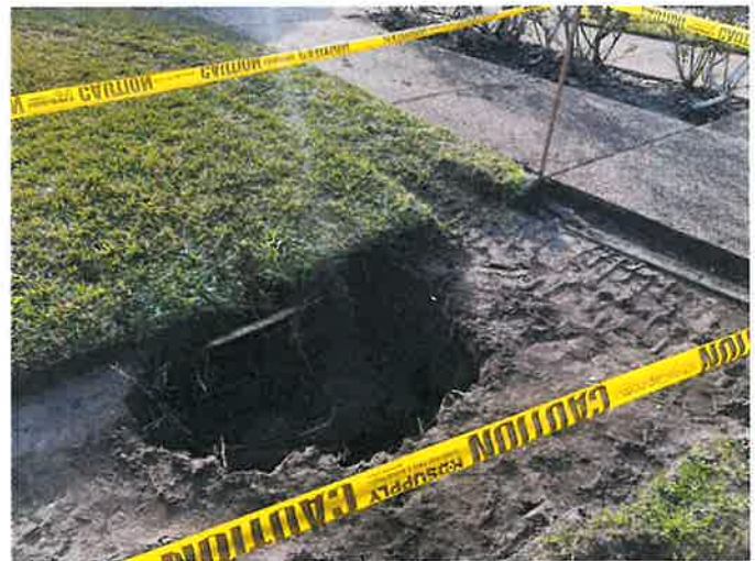
*Above Photo 0251 Void Found Underneath Sidewalk (January 2020)
