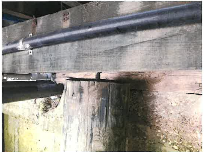
*Above Photo 2448 Timber Pier and Beam Separating, No Tie-Down (May 2020)
