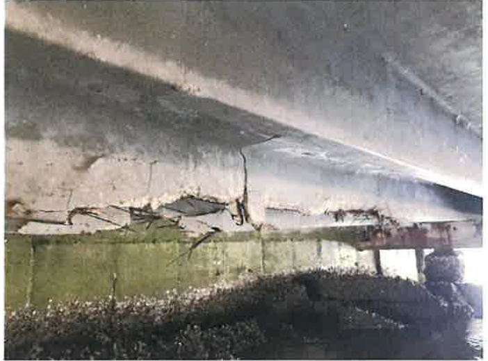
*Above Photo 2654 Deteriorated Double T Showing Severe Deflection (May 2020)
