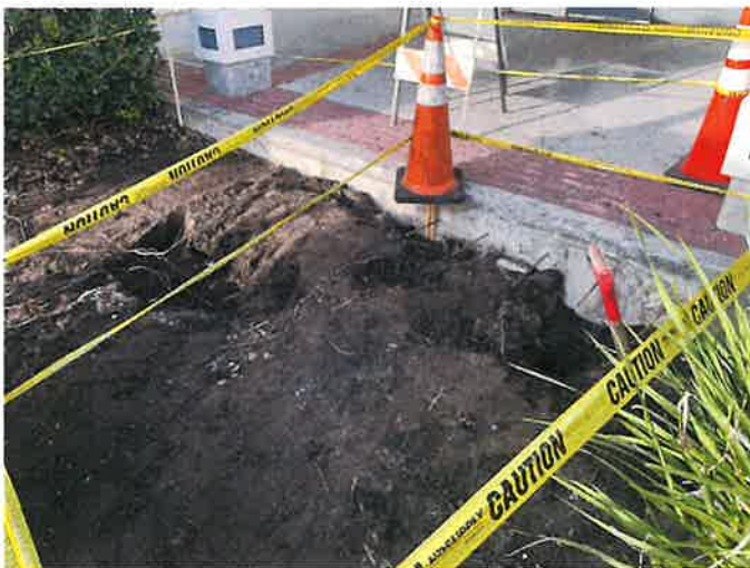
*Above Photo 0250 Void Found Underneath Sidewalk (January 2020)
