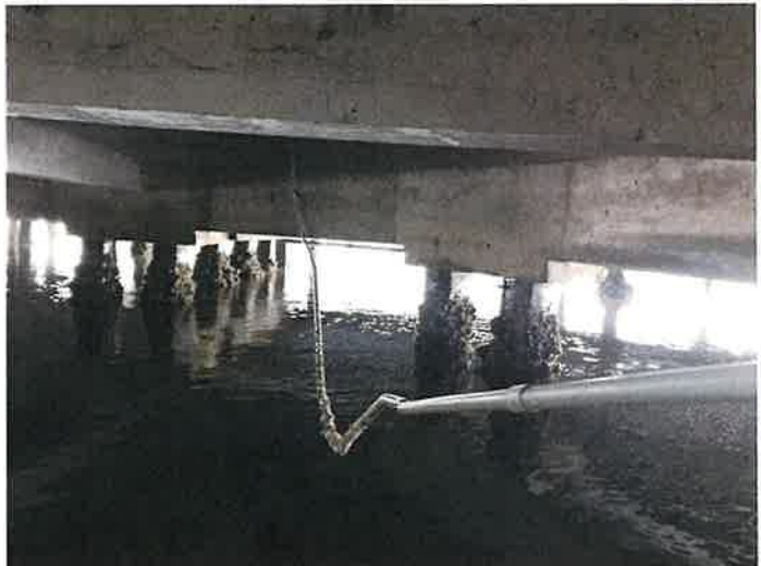
*Above Photo 2619 Unsupported and Broken PVC Conduit (May 2020)
