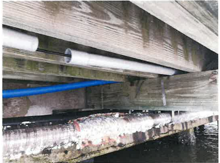
*Above Photo 2515 PVC Conduit Separated Exposing Wire (May 2020)
