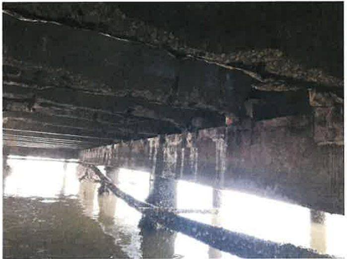
*Above Photo 2569 Hose Supports Have Deteriorated and Starting to Fail (May 2020)
