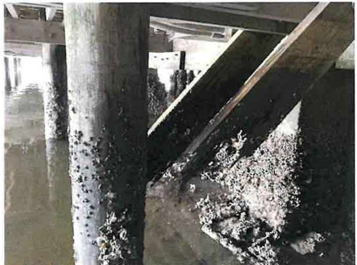
*Above Photo 2995 Rotted Timber Cross Bracing (May 2020)
