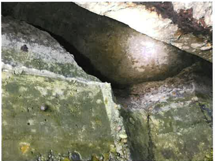
*Above Photo 2894 Water Droplets on Concrete Deck (May 2020)
