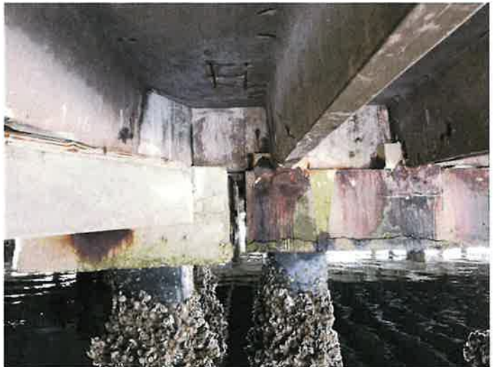
*Above Photo 2799 Deterioration of Metal Plates and Concrete Cap (May 2020)
