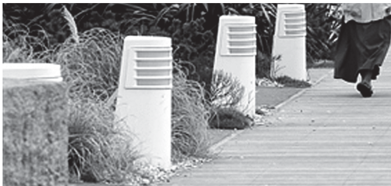
(fig. 5.20) Bollard type lights along pedestrian path.
