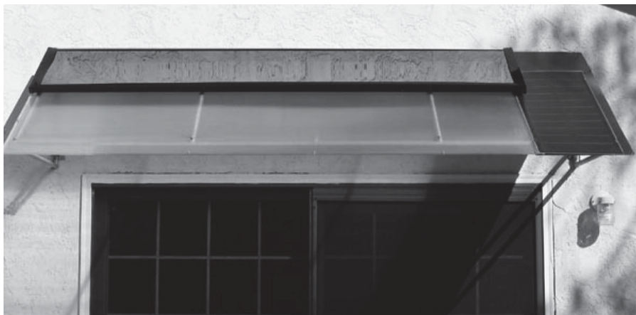
(fig. 5.19) Photovoltaic panels integrated into an awning.
