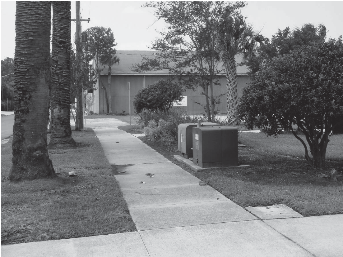
(fig. 3.10) Electrical equipment in need of additional screening.
