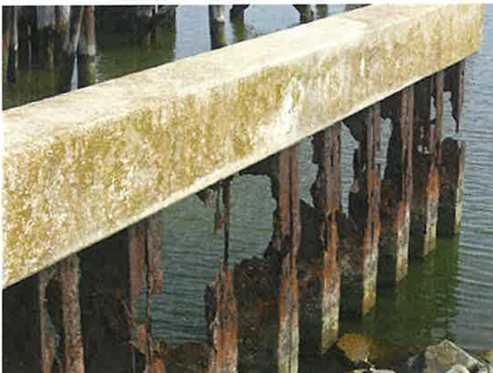
*Above corroded steel sheet pile
