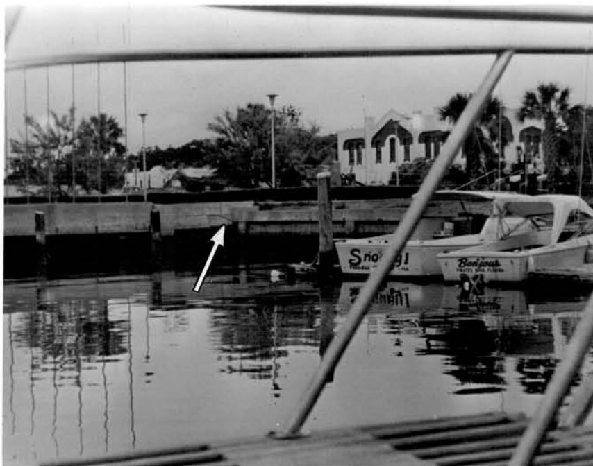
Fig. 9 Settlement and Cracking has occurred in the Portion of the Bulkhead visible in the Center of the Photograph (arrow)
