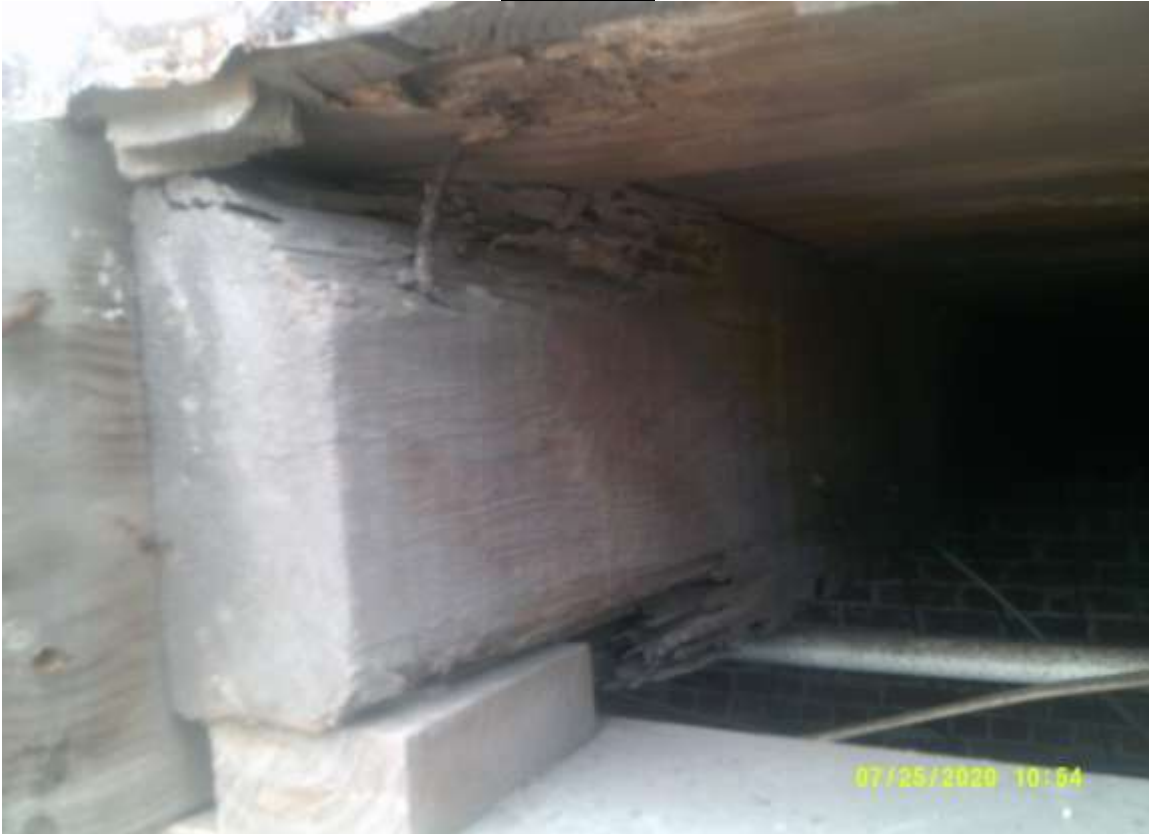
R5 NORTH BUILDING END - ROTTEN FLOOR JOIST 08/20/2021
