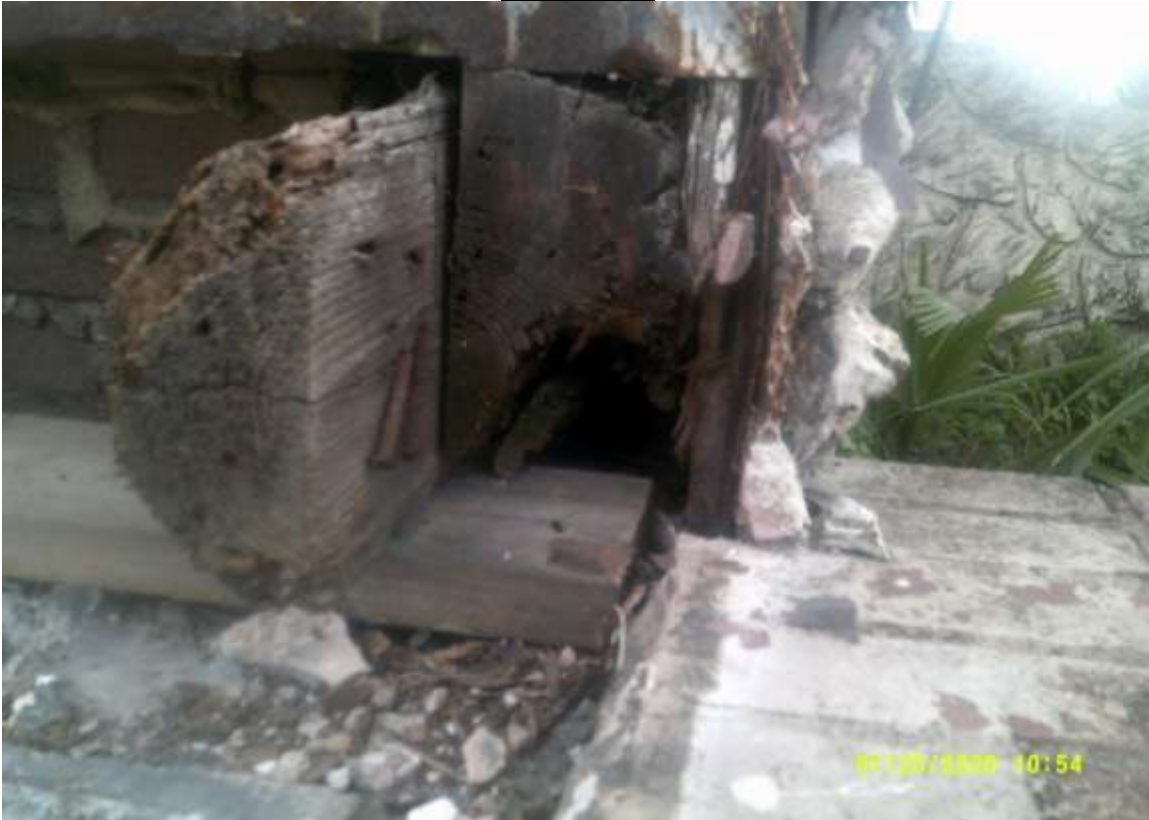
R3 NW BUILDING CORNER - ROTTEN FLOOR JOIST 08/20/2021
