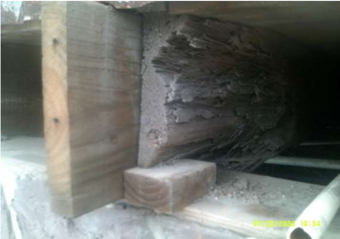
R6 NORTH BUILDING END - ROTTEN FLOOR JOIST 08/20/2021
