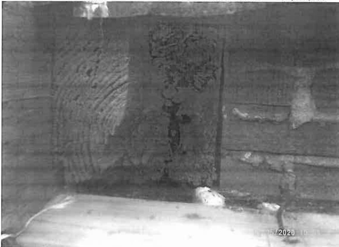
R4 NORTH BUILDING END - ROTTEN FLOOR JOIST 08/20/2021
