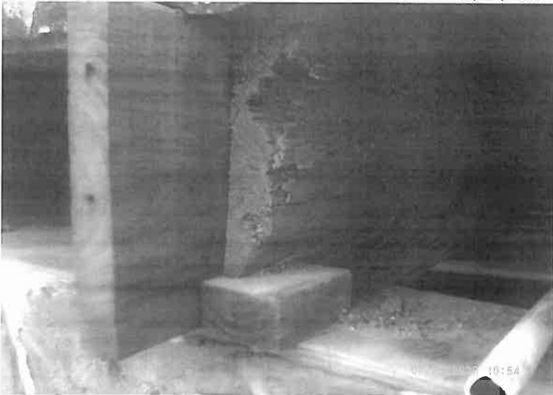
R6 NORTH BUILDING END - ROTTEN FLOOR JOIST 08/20/2021
