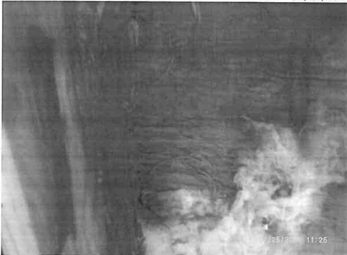
R10 ROTTEN WALL - SAMPLE LOCATION B-2 08/20/2021
