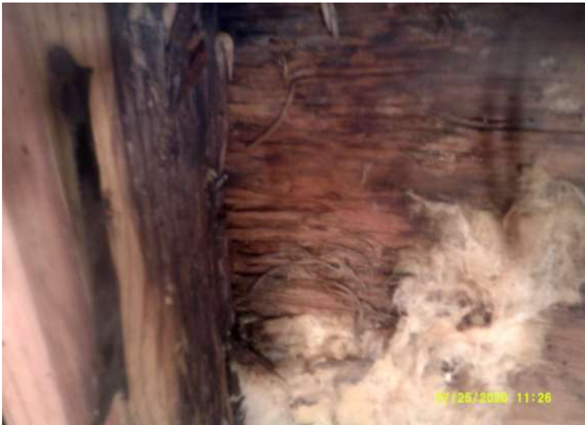
R10 ROTTEN WALL - SAMPLE LOCATION B-2 08/20/2021
