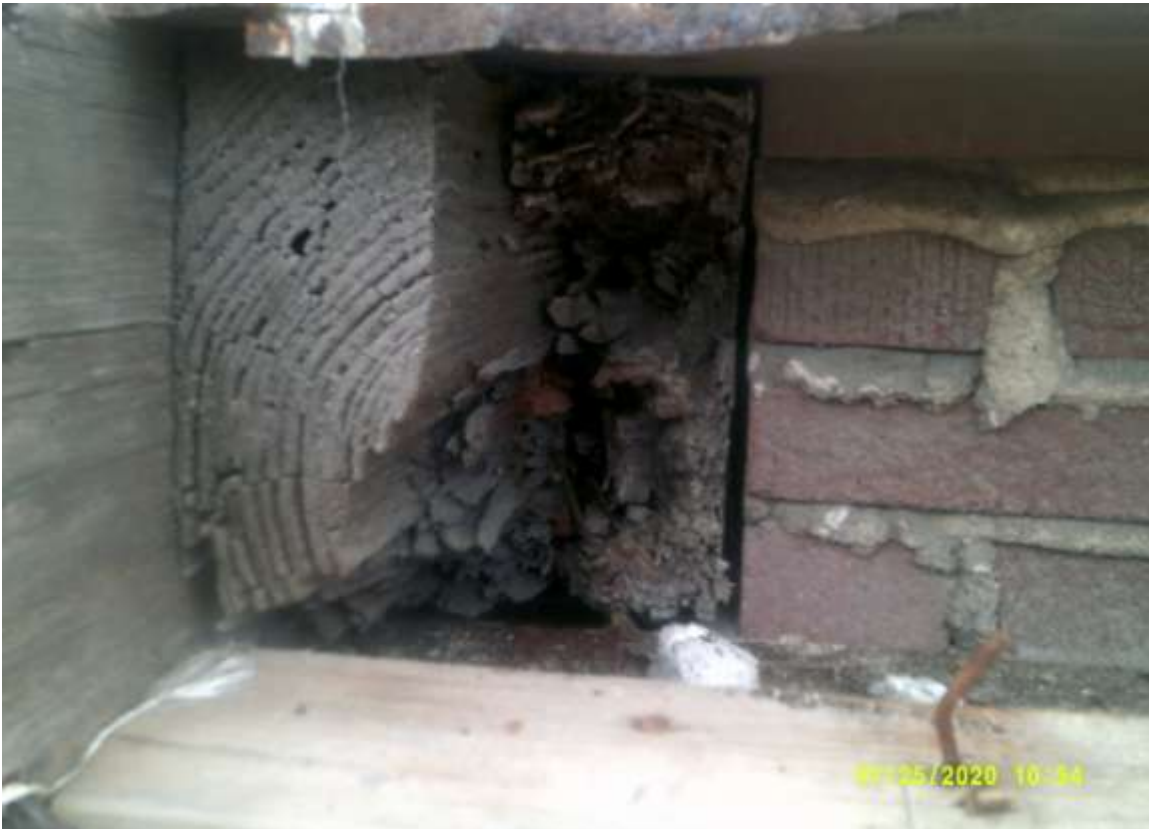
R4 NORTH BUILDING END - ROTTEN FLOOR JOIST 08/20/2021
