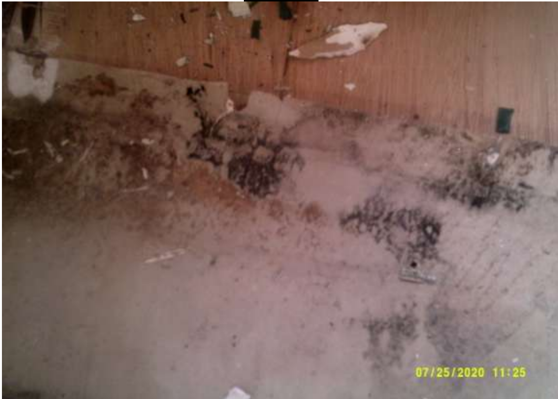
R9 ROTTEN WALL WITH MOLD/FUNGI SAMPLE B-1 08/20/2021
