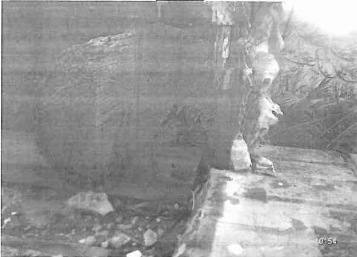
R3 NW BUILDING CORNER - ROTTEN FLOOR JOIST 08/20/2021
