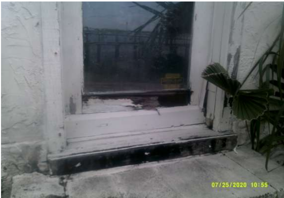
R14 WEST DOOR - ROTTEN WOOD 08/20/2021
