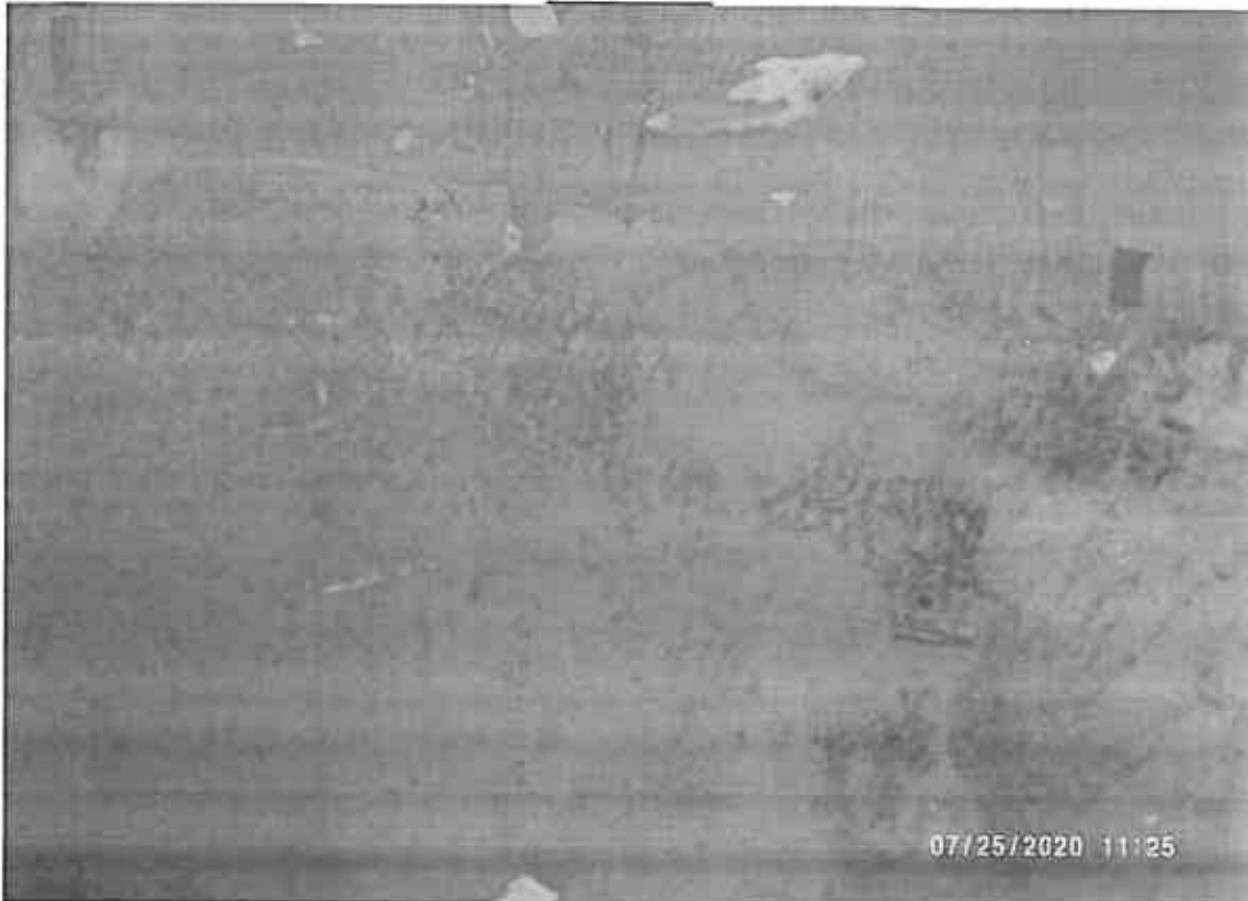
R9 ROTTEN WALL WITH MOLD/FUNGI SAMPLE B-1 08/20/2021
