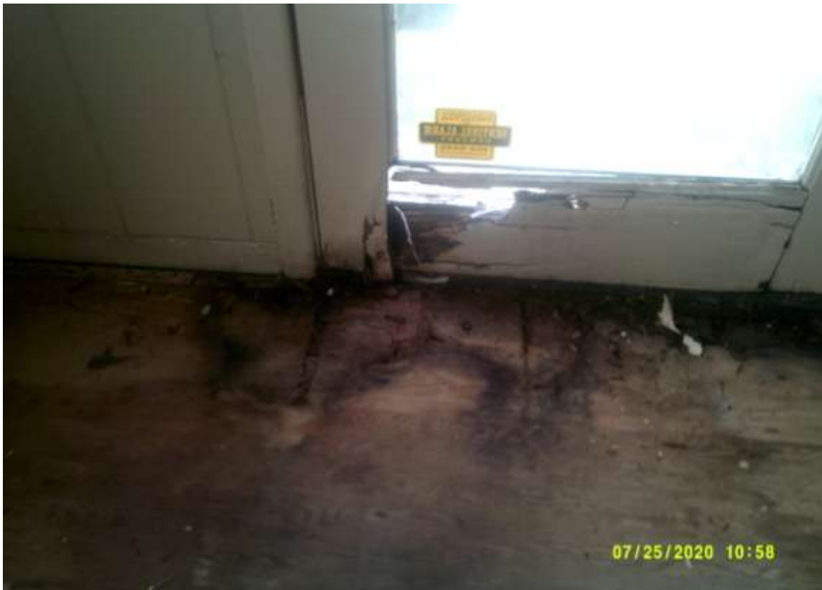
R8 ROTTEN DOOR AND FLOORING 08/20/2021
