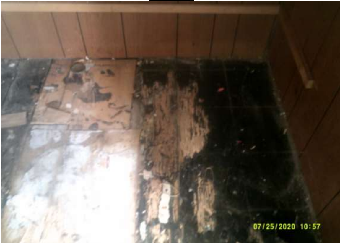
R7 ROTTEN WOOD FLOORING - OFFICE 08/20/2021
