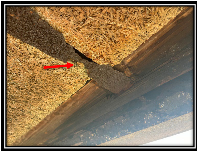
Deck Support Tee Corrosion-Typical
