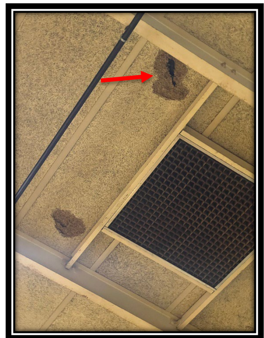
Roof Deck Staining/Holes-Interior-2
