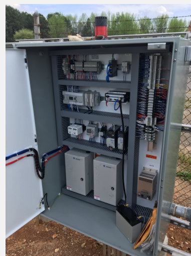
Lift Station SCADA Panel
