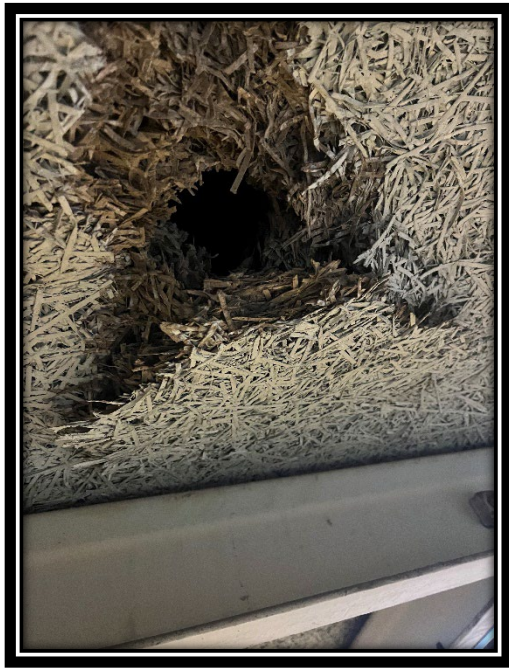
Staining/Hole in Deck – Interior-1
