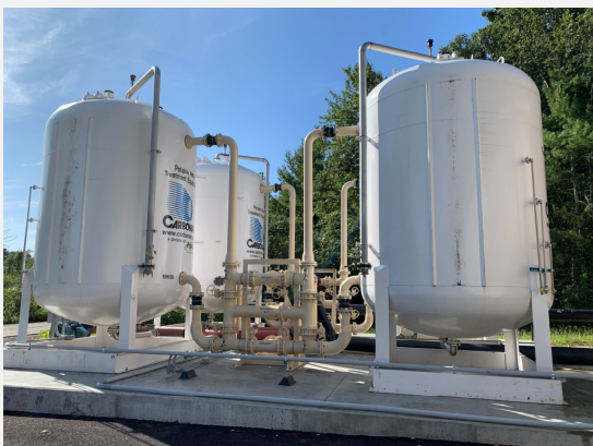
Hudson, MA PFAS Removal System
