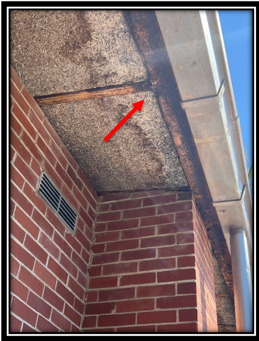
Corroded Eave/Tee – (Upper South Side)
