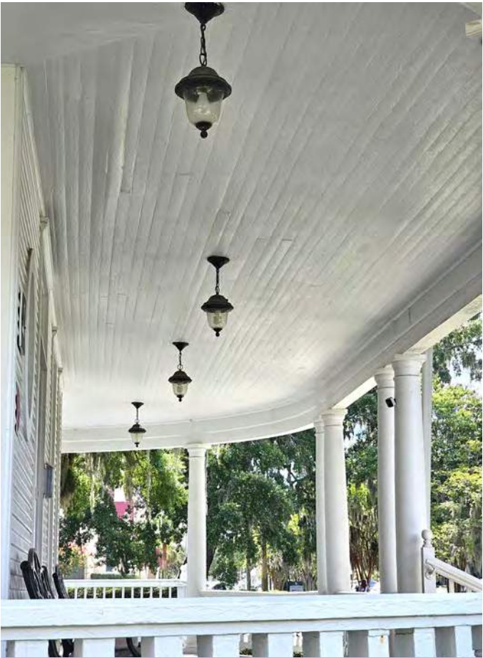
PORCH LIGHT FIXTURE 603 Centre Street
