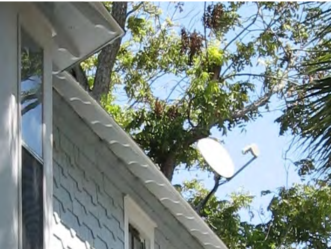
DISH ANTENNAE PLACEMENT 214 South 7th Street
