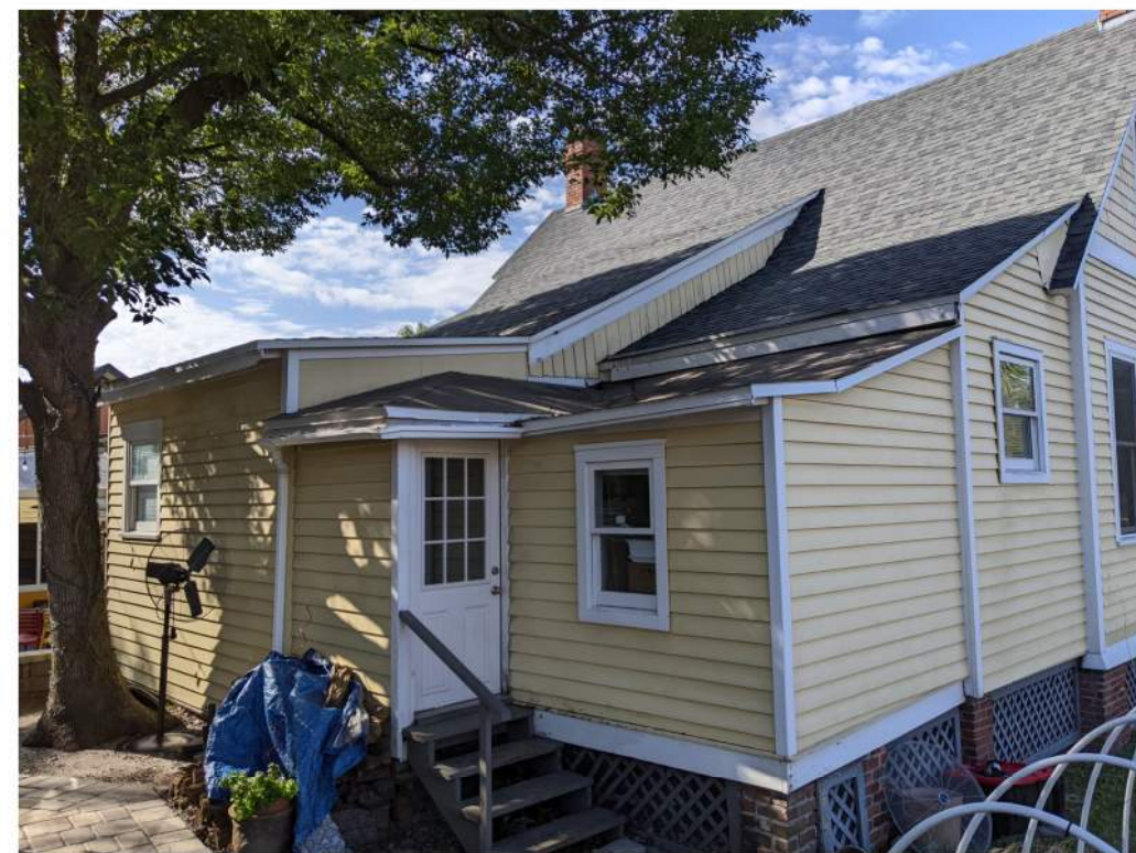
VIEW FROM NE PROPERTY CORNER, CLOSE UP SAME NOTES FROM ABOVE. THE VERTICAL T-11 INFILL IN THE GABLE IS COMPROMISED AND WILL REQUIRE REPLACEMENT WHEN THE WALL IS RECONSTRUCTED.
