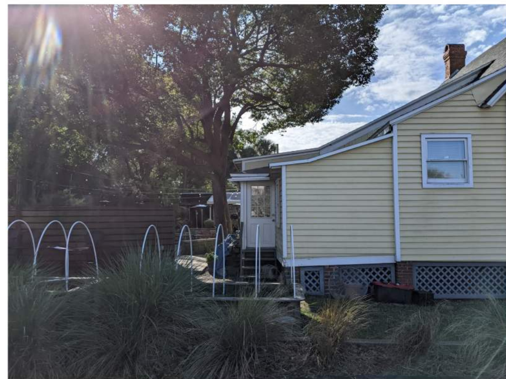
VIEW FROM NORTH PROPERTY LINE MORE OF A DIRECT VANTAGE SHOWING THE SHINGLE ROOFS AND EAVES, TRIM AND SAGGING FLOOR CONDITION
