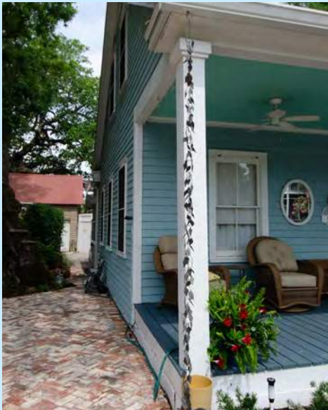
RAIN CHAIN 111 South Sixth Street
