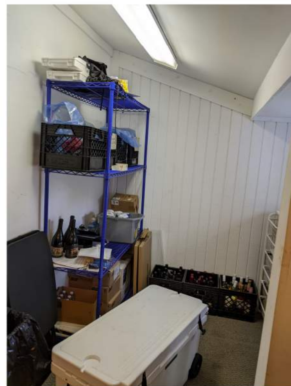
INTERIOR VIEW FROM INSIDE STORAGE REFERENCE PHOTO SHOWING SAGGING FLOOR TO THE RIGHT
