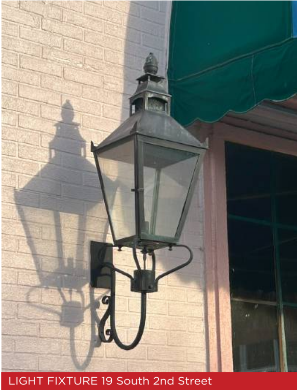
LIGHT FIXTURE 19 South 2nd Street 19th Century Carriage Light
