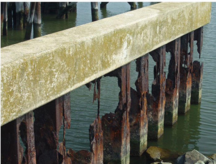
*Above corroded steel sheet pile
