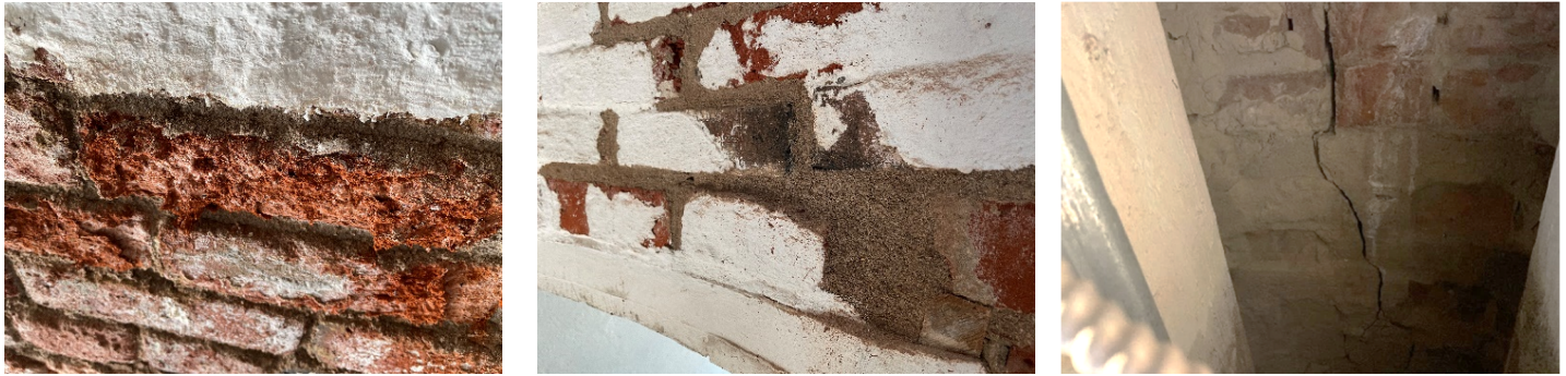
Photo 4, 5 and 6 (Left to Right): Typical spalled brick condition and efflorescence near base of lighthouse interior; previously repointed mortar joint with newer mortar material; vertical crack within weight box at interior masonry wall.
