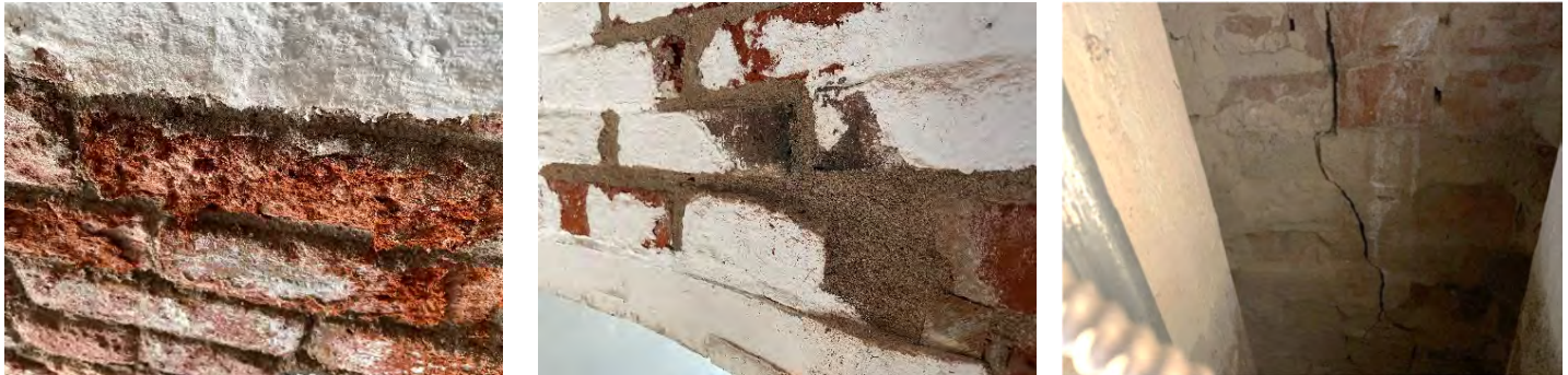
Photo 4, 5 and 6 (Left to Right): Typical spalled brick condition and efflorescence near base of lighthouse interior; previously repointed mortar joint with newer mortar material; vertical crack within weight box at interior masonry wall.
