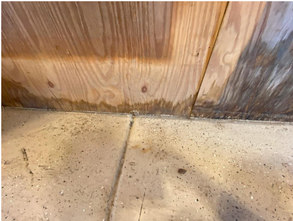
Water wicking up the interior plywood occurs the entire perimeter
