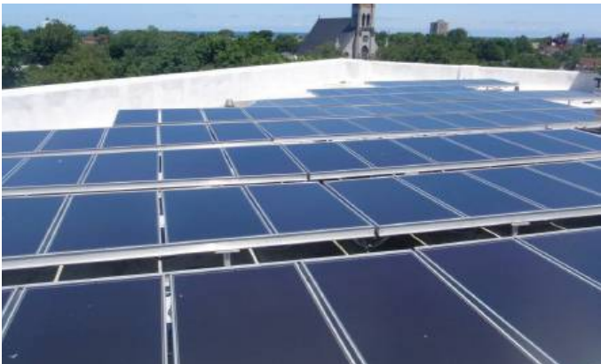
SOLAR PANELS EXAMPLE
