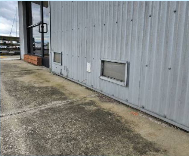
FLOOD VENT 204 South 6th Street
