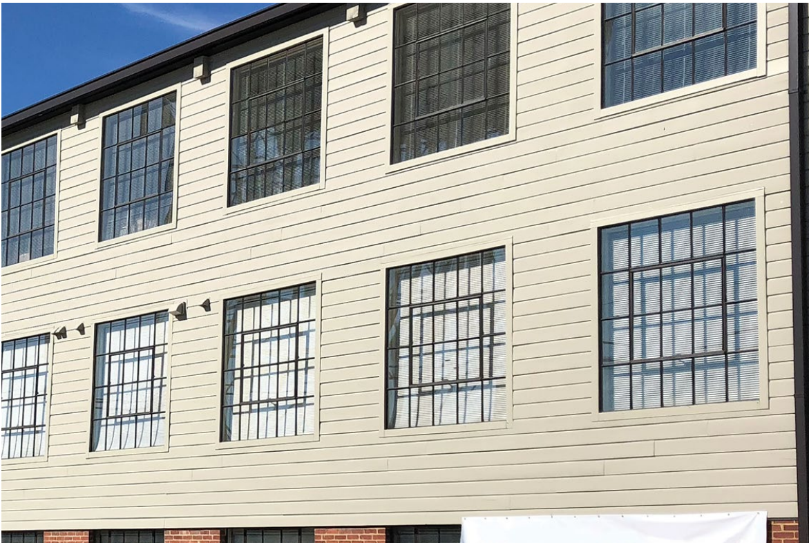
Figure 21. A mineral polymer composite siding was available in the profile very similar to the historic siding. The replacement siding was used where the original material was almost completely missing beneath a more modern covering. Areas where the original wood were largely intact were replaced with matching wood to sustain more of the material integrity of the building. Photo: Belk Architecture.
