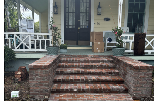
D3. EXISTING BRICK STEPS IN WEST ELEVATION
