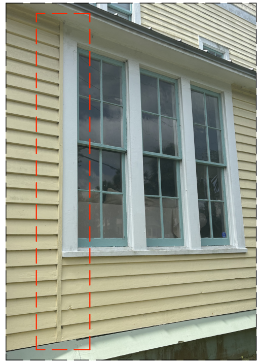
D1. EXISTING MOLDING ON NORTH ELEVATION TO THE BREAKFAST ROOM ADDITION
