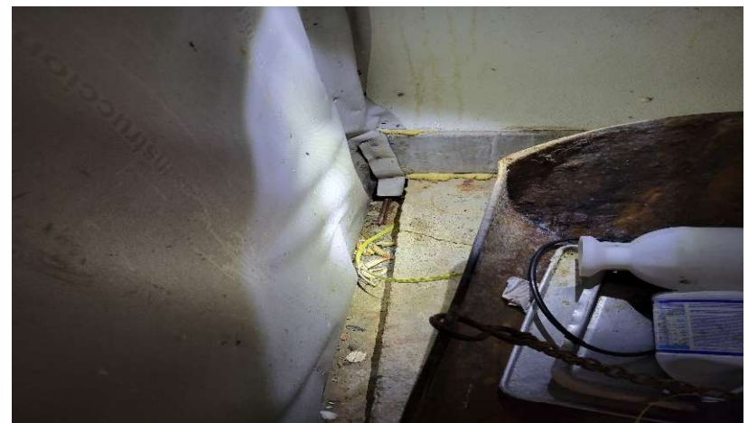
Fish Room – Separation Btwn North Wall & Floor Slab
