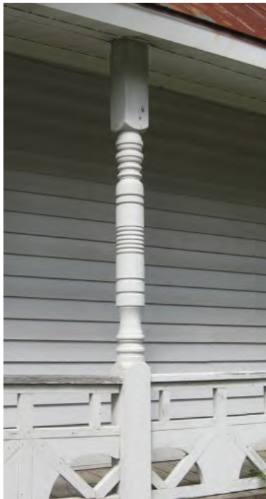
Preserve and maintain porch elements such as this column at 107 Estrada Street.
