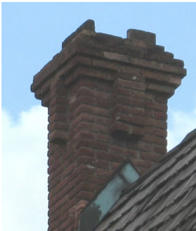
Original corbelled brick chimneys should be maintained and repaired as needed (910 San Fernando Street).
