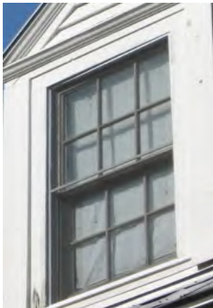
Below: The window screens are difficult to see, allowing for full view of the original six-over-six wood sash window (902 Ladies Street).
