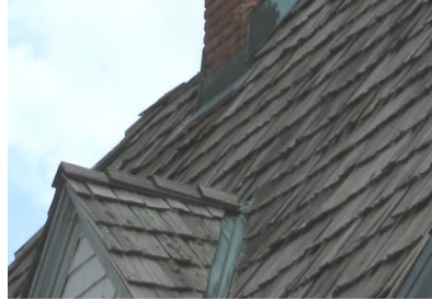
The use of wood shingle roofs as a replacement material is appropriate for contributing dwellings (910 San Fernando Street).
