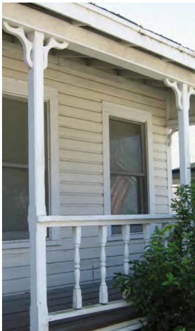
Simple porch columns and railings are recommended for vernacular dwellings such as on this rebuilt porch (714 San Fernando Street).
